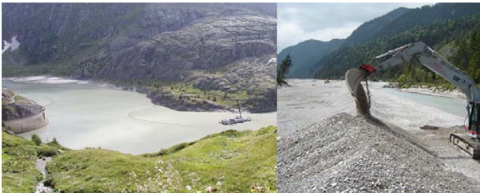
Photo 9 Excavation activities in reservoirs: Suction dredger and floating pipeline at the pilot action Margaritze (left) and conventional hydraulic excavator at Sylvenstein (right) (ALPRESERV project).
