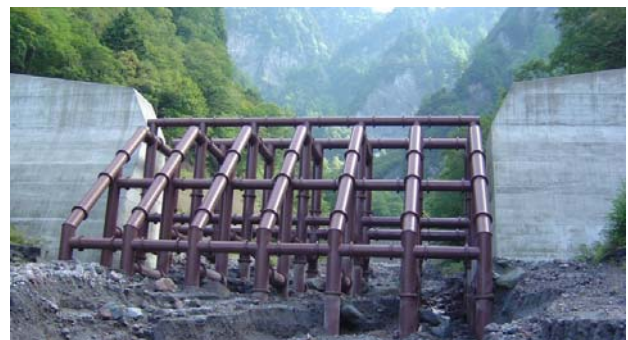
Photo 2 Slit check dam from steel pipes http://www.dpri.kyoto-u.ac.jp/rcfcd/sabo/index.htm
