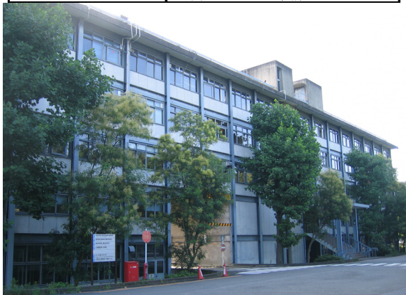
Photo 1 The object building before the reinforcement (Uji campus main research building, east building)
