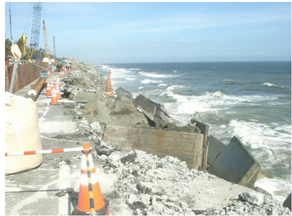
Photo. 3 Storm-induced damage to a stretch of retaining wall of the Seisho Bypass (photograph 16 September 2007)
