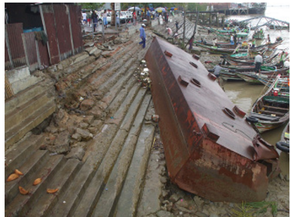
Photo 5 Broken pontoon on seawall
