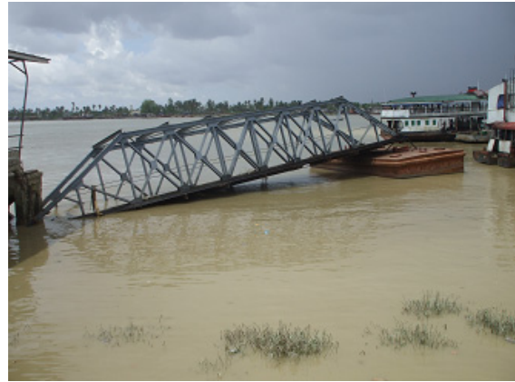
Photo 4 Damage of connection bridge
