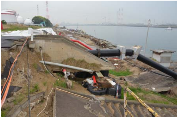
Figure 22 Damaged embankment in Kajima port
