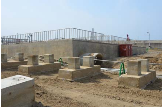
Figure 21 Uplift of the reserve tank in Hitachinaka electric power station.
