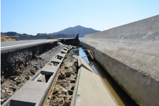
Figure 3 Damage to coastal levee in Kesen'numa
