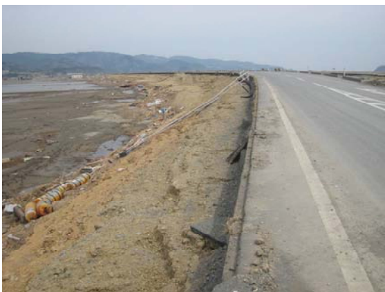
Figure 13 Washed embankment near the Shin Kitakami River
