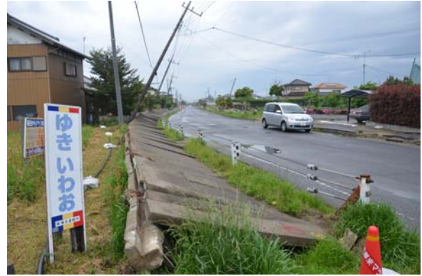
Figure 23 Inclined electric pole and uplifted lids of drain in Hinode cho, Itako city.
