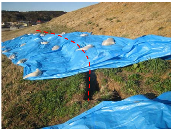
Figure 17 Semi-circular crack observed in the embankment of the Kitakami River (45.5k).
