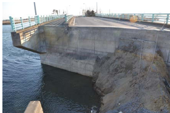
Figure 15 Lost embankment of Jokawa bridge.
