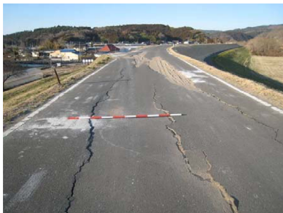
Figure 18 Longitudinal cracks at the top of the embankment of the Kitakami River (45.5k).
