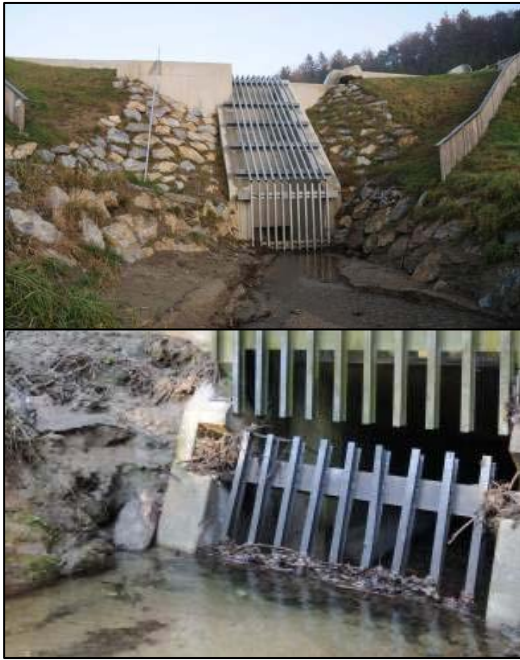
Fig. 5 screens installed at the inlet of bottom outlet
