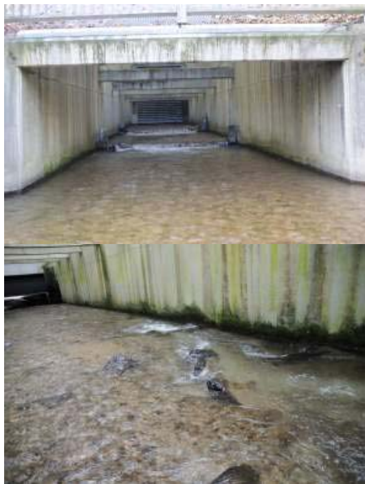
Fig. 6 Natural fish passages in bottom outlet approach channel equipped by stones and sunlight
