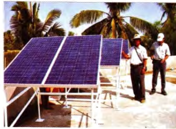
Solar Power system
