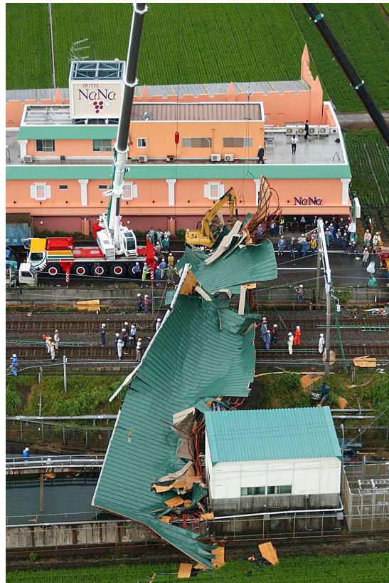
Photo 1 Blown roof of a hotel onto JR track. (Yomiuri news paper, 2004/6/22)
