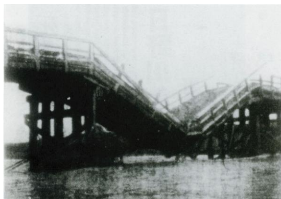
Photo 4 The Ichido Bridge was damaged by Typhoon Isewan (source: Shiga Prefecture homepage)
