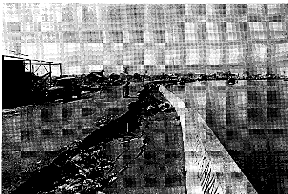
Fig. 9 Failure of river protection walls at Lampulo
