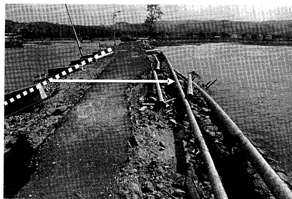
Fig. 11 Minor damage to the embankment for pipelines at Malahayati. Pipelines were dislocated.
