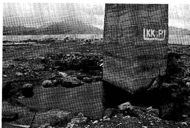
Fig. 5 Erosion behind the monument located at Ulee Lheue
