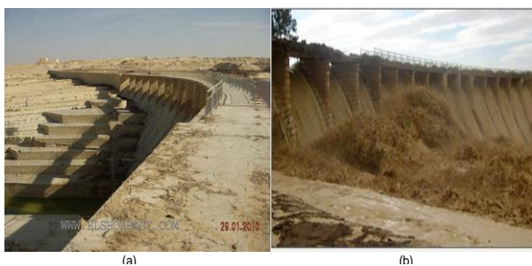
Fig. 9 El-Rawafaa Dam before the flash flood (a), and during the flash flood event in January, 2010.
