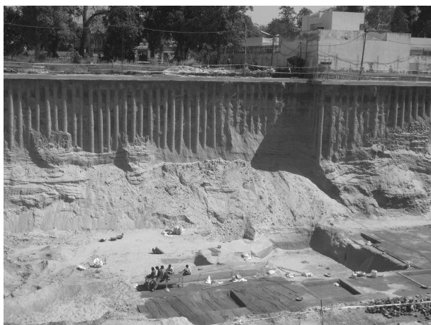
Fig. 3 Shoring piles prior to failure
