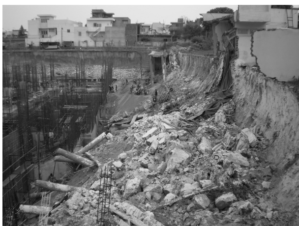
Fig. 4 Post failure conditions
