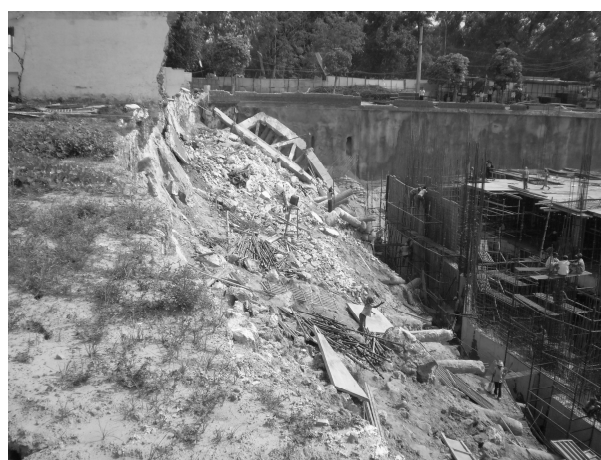
Fig. 6 Another view of post failure conditions
