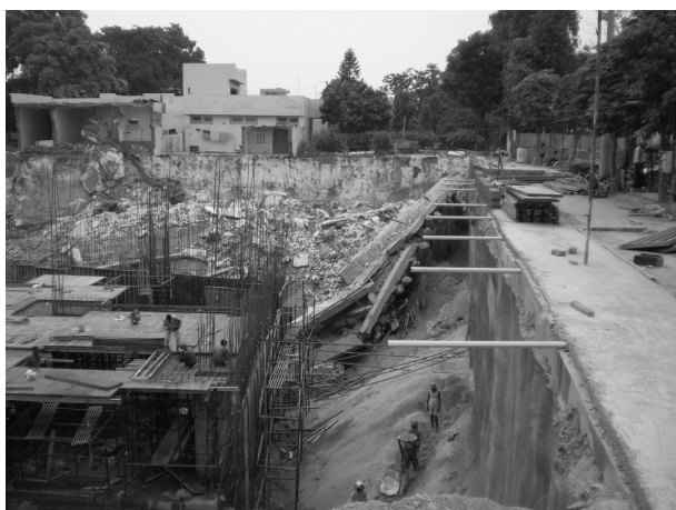
Fig. 5 Front view of shoring piles post failure
