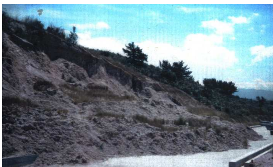
Fig.1 Picture of the slope failure
