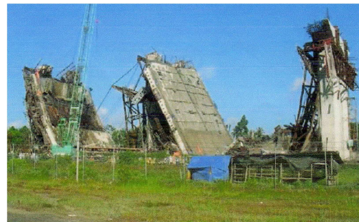
Fig.14 Collapsed concrete girder
