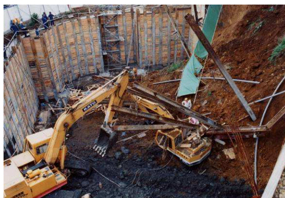
(b) The scene of the collapse accident (from north side)
