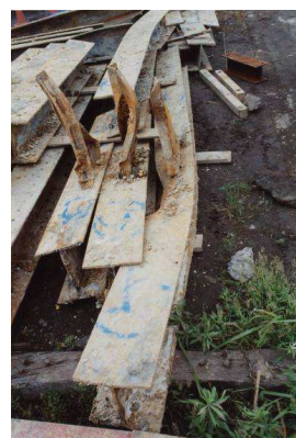
(c) Damaged H- steel for anchor head Fig. 3 The scene of the collapse accident
