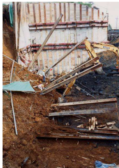
(a) The scene of the collapse accident (from south side)
