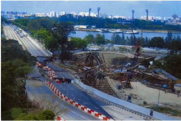
Figure 17 Nicoll Highway subway construction collapse
