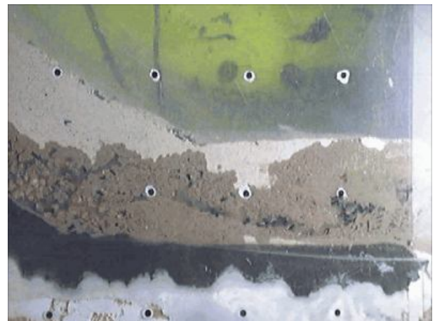
Figure 6 Trace of stored water escaping beneath fast flowslide in dense CDG (Wong, 2003)
