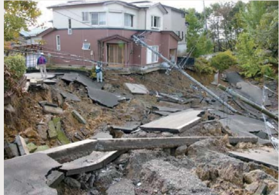
Earthquake-induced landslide after the 2004 Niigata Prefecture Earthquake (Professor Kamai, Kyoto University, Japan)
