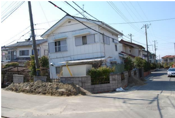
Photo 1 Settlement and tilt of residential house in Chiba city
