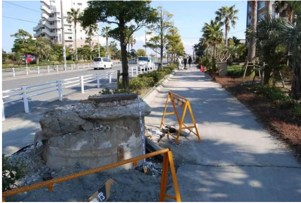
Photo 2 Uplift of manhole and settlement of pavement in Urayasu city
