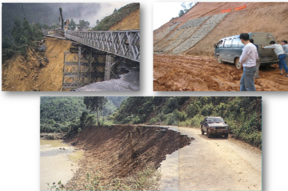
Landslide along Ho Chi Minh National Highway
