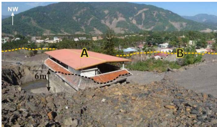
Fig. 8 Photo of the buried houses where the photo was taken toward northwest from the location marked A in Fig. 1. At the location A, from the trace on the wall, the flow depth of debris flow is about 6m at least. The deposition depth of the debris flow front is about 2~3 m, as shown at the location B.
