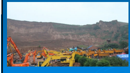
Baqiao landslide in Shaanxi Province triggered by rainfall
