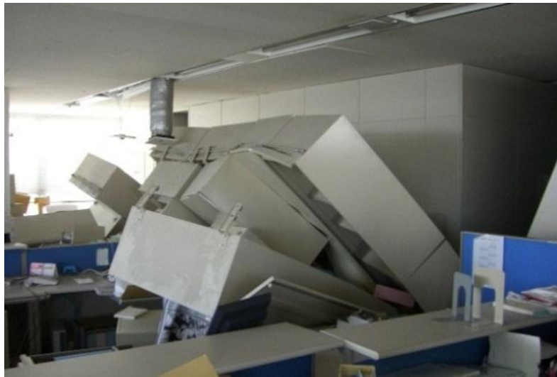
Figure 2.1 Contents damage inside the structure
