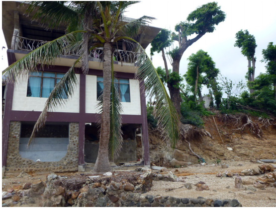
Photo 4 Damaged building and scoured cliff at Pa-on beach resort in Estancia. Clear water mark was observed inside the room of second floor. Stone walls of the first floor are collapsed by wave force.
