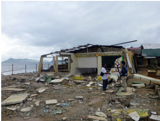
Photo 5 Collapsed walls and roofs of Mabuhay elementary school in Estancia.
