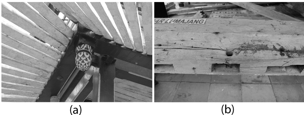
Figure 10. (a) The outermost band of rectangular beams, (b) mortises beam, where a series of rafter will be inserted.
