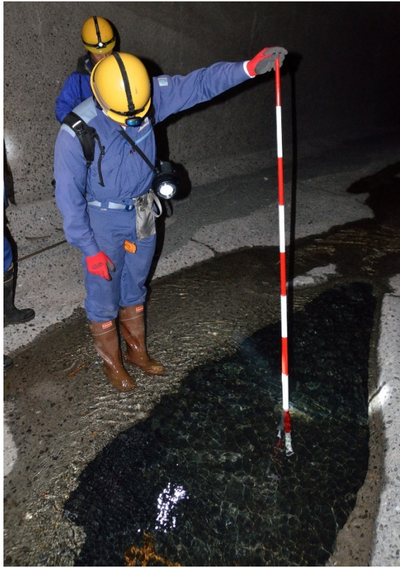
Fig. 1 Concrete invert abrasion at Asahi SBT, Japan (photo: C. Auel).
