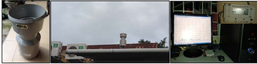
(a) Rain gauge (b) Installed on the house's roof (c) Recorder connected with PC
