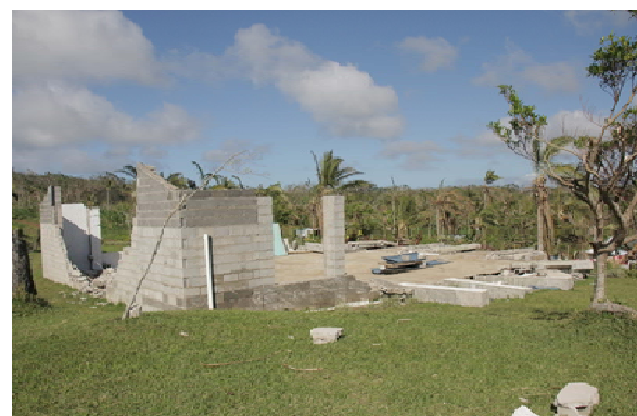
Figure 5. Collapsed church building in Green Hill.
