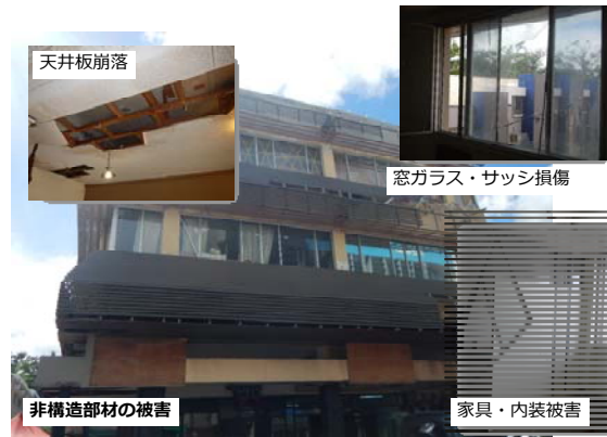
Figure 3. Damages to an office building in the capital, Port Vila.
