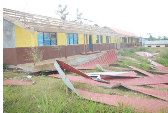
Figure 4. Damages to a school building located in the middle of Tanna island.
