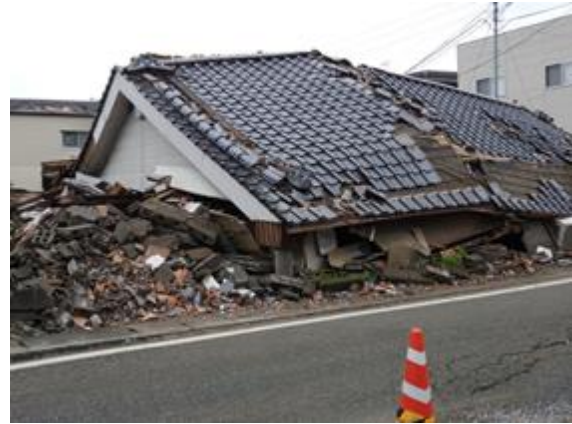
Fig. 3 The totally collapsed wooden house
