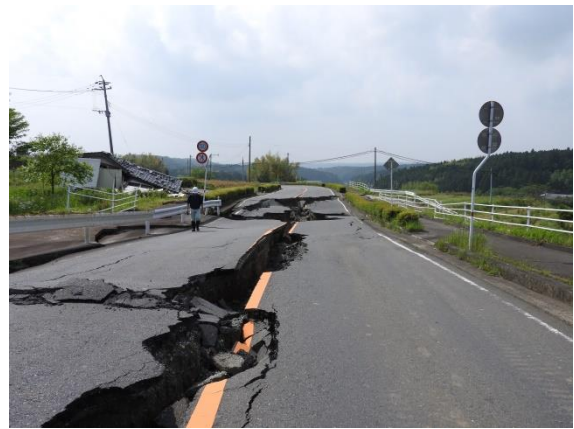
Fig. 17 The collapsed road
