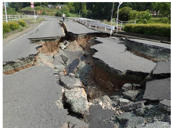
Fig. 18 The collapsed road
