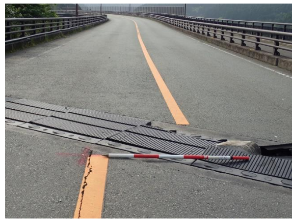
Fig. 23 Lateral displacement of the bridge to the north direction
