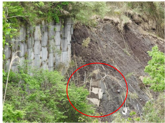
Fig. 35 The collapsed Terre-Armee retaining wall
