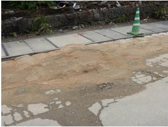
Fig. 11 Sand boiling due to liquefaction
