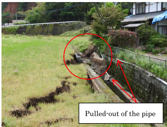
Fig. 16 The collapsed retaining wall on the fault and pulled-out of the water pipe
