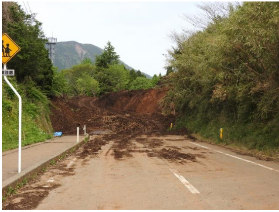
Fig. 33 400m away to the downstream preventing from the road use
