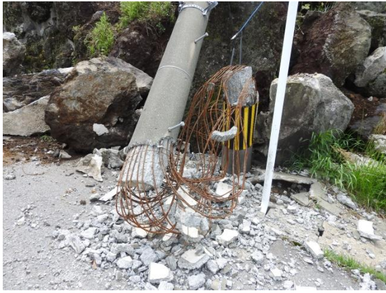
Fig. 37 The greatly bending electric pole
