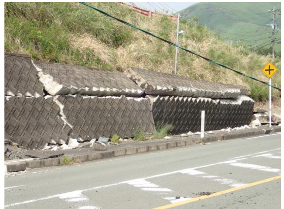
Fig. 28 The broken retaining wall on the fault
