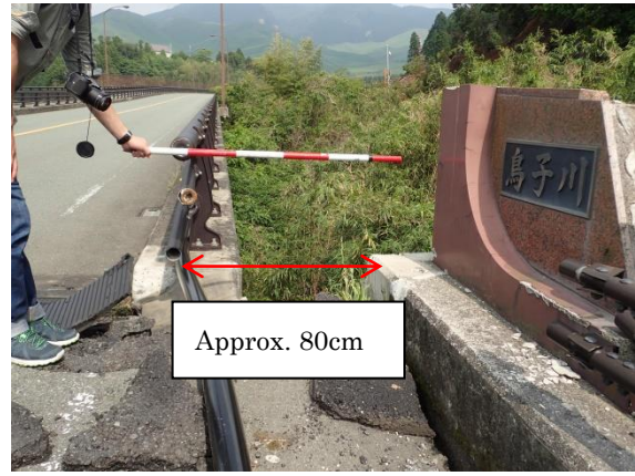
Fig. 22 Lateral displacement of the bridge to the north direction
