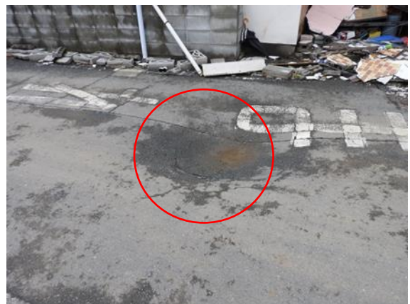
Fig. 9 Settlement of the road due to liquefaction
