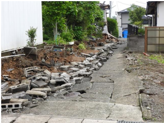
Fig. 12 The collapsed block retaining wall
