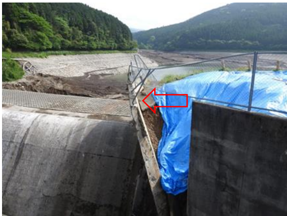
Fig. 25 The broken retaining wall
