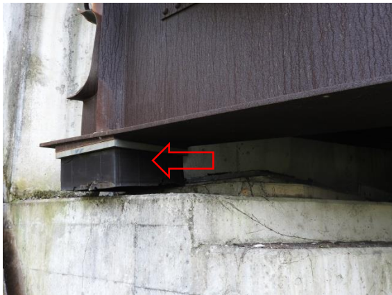
Fig. 21 The broken rubber bearing
