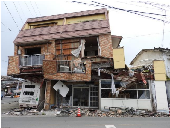
Fig. 6 The damaged three-stories buildings with the broken column at the second floor
