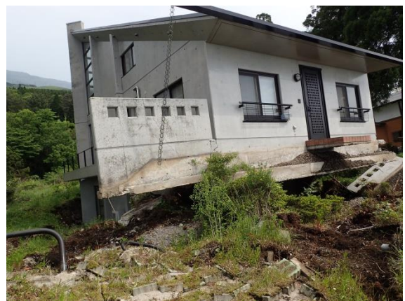
Fig. 36 The inclined house due to the collapse of the Terre-Armee retaining wall
