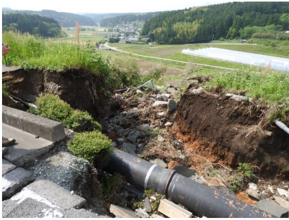
Fig. 20 Soils were washed out due to the leaked water from the broken water pipe.
