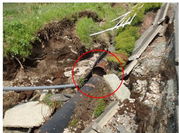
Fig. 19 The pulled-out pipe
