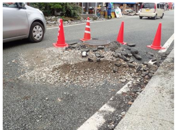
Fig. 10 Up-lift of the manhole due to liquefaction
