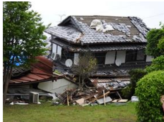
Fig. 4 The partly collapsed wooden house
