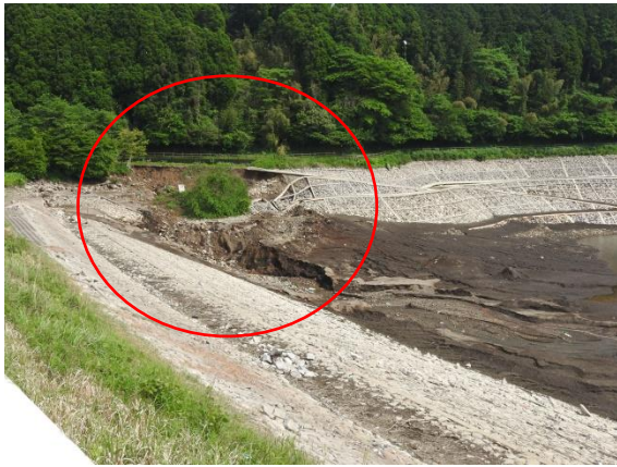
Fig. 24 The broken slope of the dam reservoir
