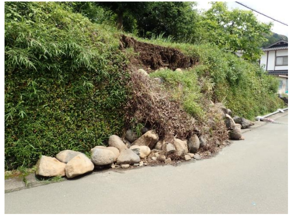
Fig. 13 The collapsed stone retaining wall
