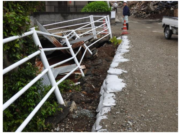
Fig. 8 The inclined fence following the spreading of the embankment
