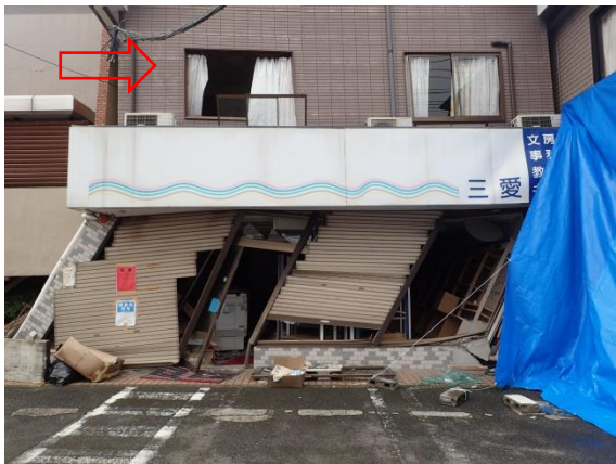
Fig. 7 The inclined house leaned by the left adjacent buildings
