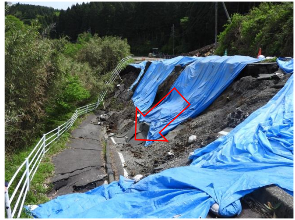
Fig. 34 The collapsed Terre-Armee retaining wall
