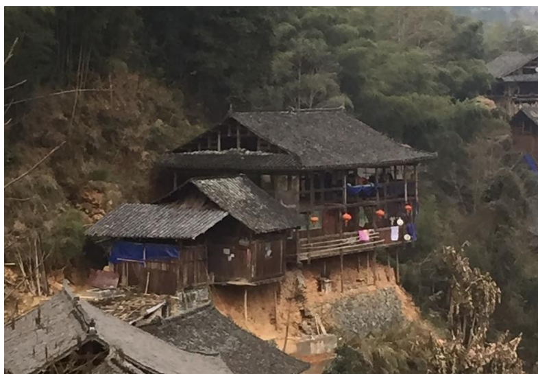
Figure 4.8 The most severely affected building, whose foundations collapsed
