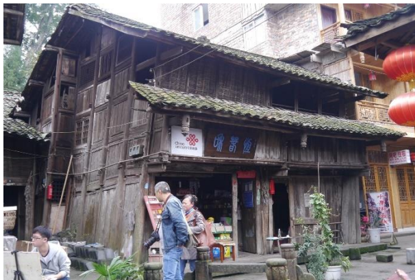
(a) Leaning building
