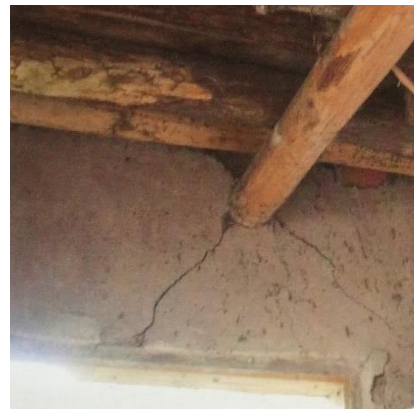
(b) Cracked backwall
