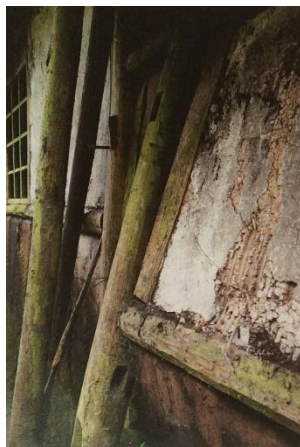
(c) Distorted wall and pillars
