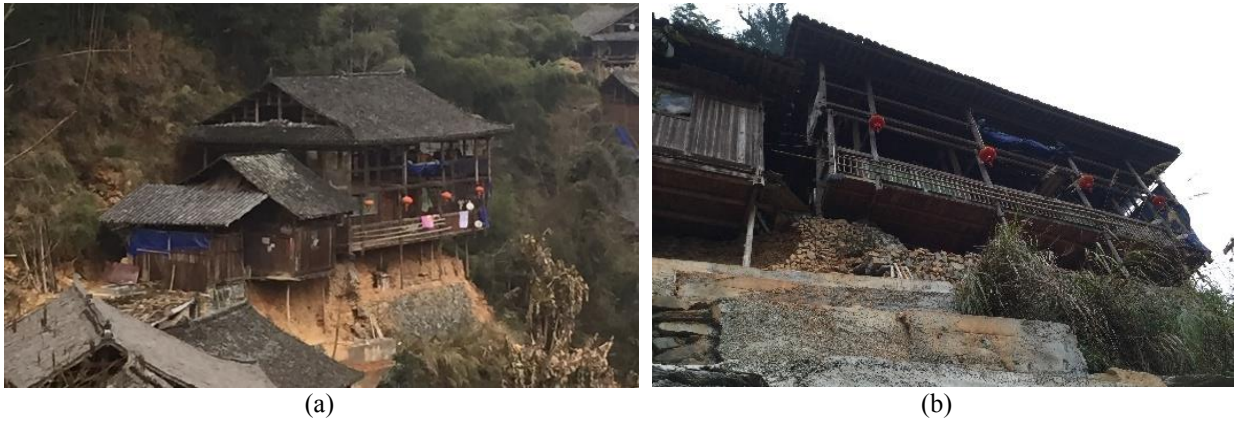
(a) The most severely affected building, whose foundations have already collapsed (b) This household was repeatedly repairing and strengthening the foundations with stone and cement
