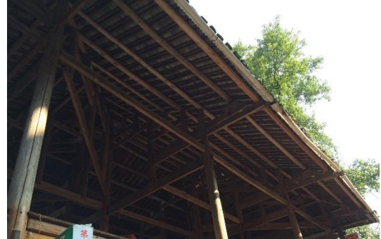
(b) Wooden roof truss and eaves without a fire-resistant coating
