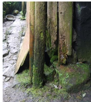
(f) Rotten pillars on spot (f)
