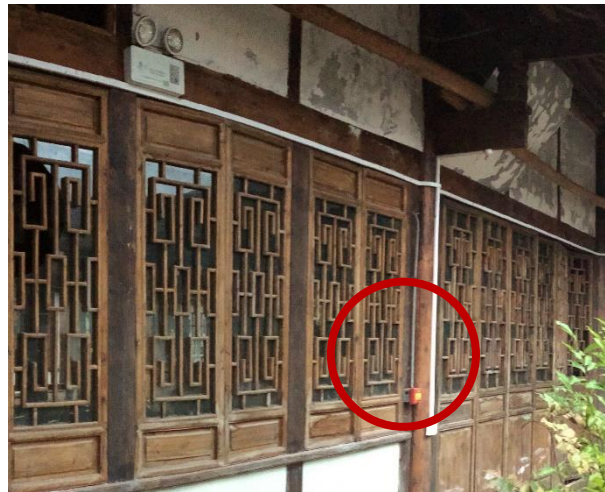
Figure 7.7 Fire alarm only assembled in the most important heritage building in Shangli Village
