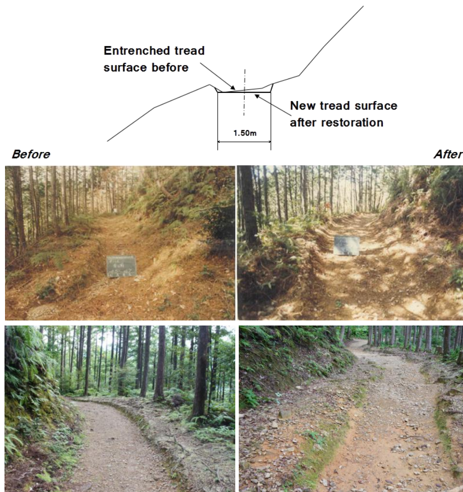
Figure 4.6 An example of the soil excavation practice in the restoration project 1978–1982. a. Upper-left, photo from the construction report that was taken before construction; b. Upper-right, photo from the construction report that was taken after construction. The sketch above the photos was drawn by the author, based on the original design graph (Photos are credited to the Local Education Office of the Hongu-District.). c. Bottom-left, photo taken by the author in 2013 at a location close to the locations of the two photos above. The sharp descent near the trail edge was used for the on-site identification of such practices; d. Bottom-right, a disturbed surface of the entrenched trail caused by lateral erosion. Photo taken by the author in 2013 near that shown in c.
