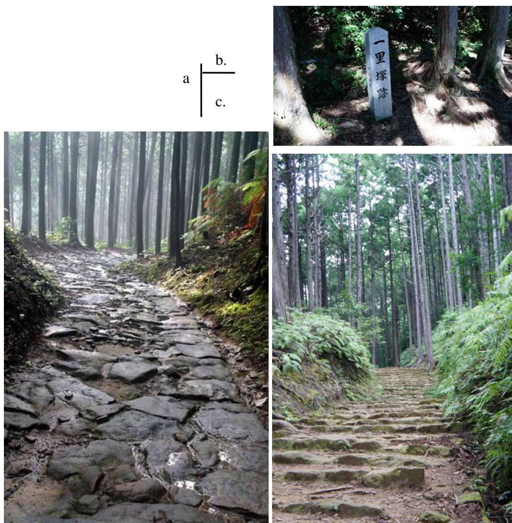
Figure 3.3 Remaining of road reparative and maintaining construction during Edo era ordered by then ruler of the Kishu Domain on Nakahechi Route for the section from Hosshinmon Oji to Kumano Hongu Taisha shrine. a. Stone-pavement; b. Relics of Ichiri zuka (milestone); and c. Stone steps.
