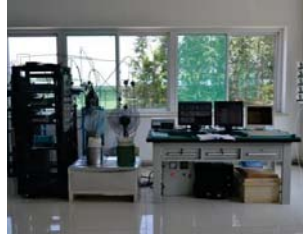
Oxygen measurement and control
