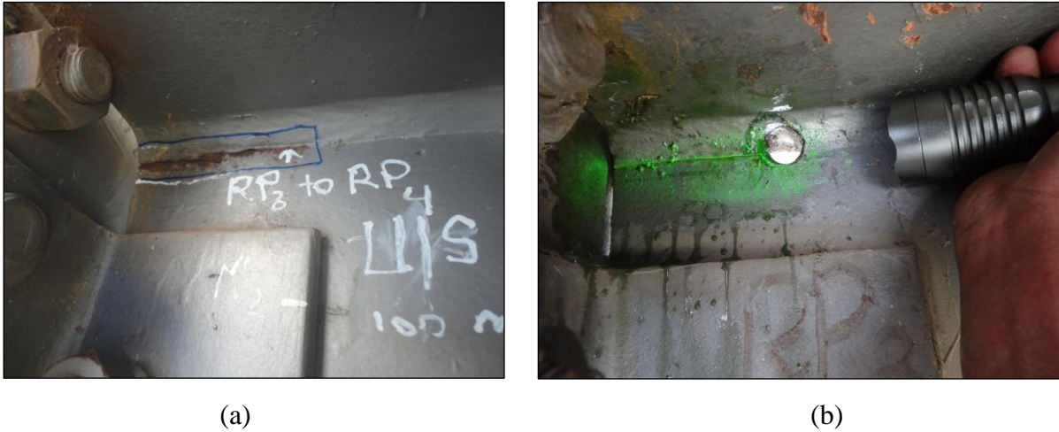
Figure 2.6: (a) Crack in the welded joint between the top flange and the web; (b) Stop hole drilled at the tip of crack.
