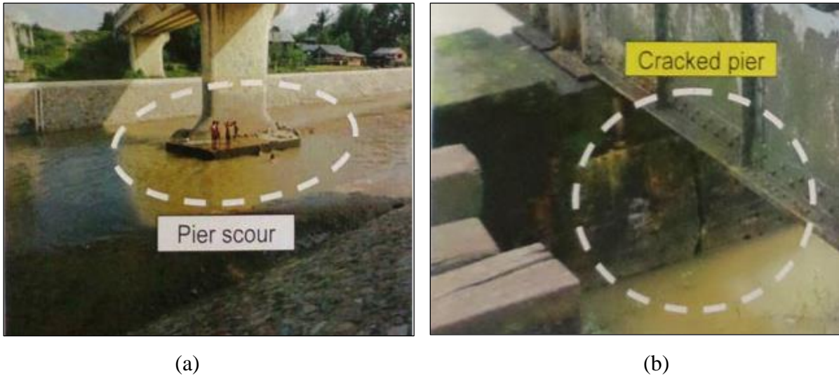
Figure 2.9: (a) Pier scouring in bridge No. 393; (b) Cracked pier in Bridge No. 21.
