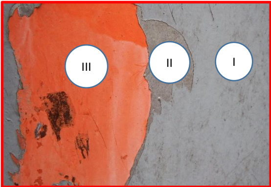
Figure 5.4: Peeling off paint layers in Maubin Bridge
