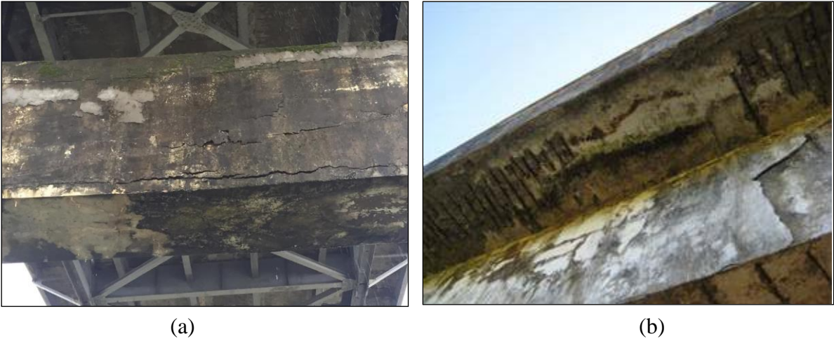
Figure 2.2: (a) Corrosion of bridge bent in Min Chaung Bridge; (b) Corrosion of bottom cover underneath the side walk in Lone Daw Pauk Bridge.
