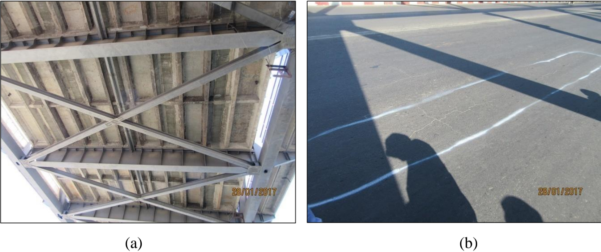
Figure 2.7: (a) Precast concrete deck slab seen from underneath the bridge; (b) Cracks in pavement on the bridge due to the deflection of precast concrete slab.
