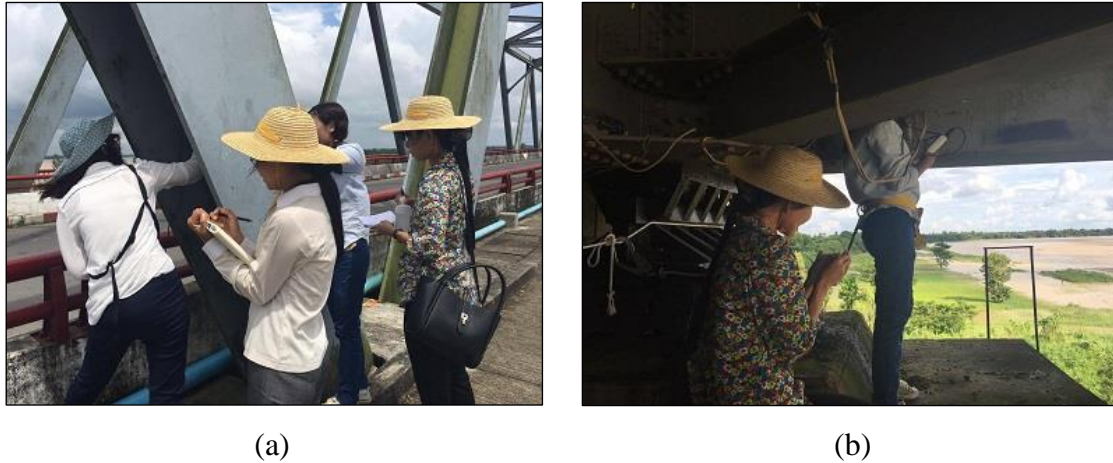
Figure 5.12: (a) Measuring member thickness by ultrasonic thickness meter; (b) Coating thickness and surface salinity measurements on pier (P4)
