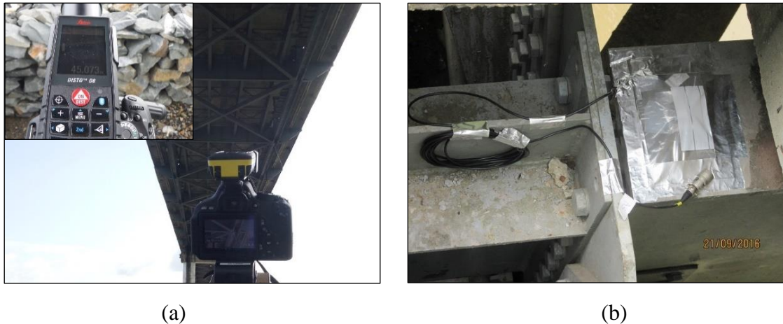
Figure 5.11: (a) Deflection measurement of location 2 from the ground; (b) Accelerator installed on the cross beam at location 3.
