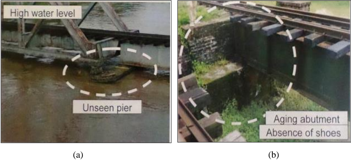
Figure 2.8: (a) Unseen bridge pier during high water level in bridge No. 111; (b) Aging abutment and absence of shoes in bridge No. 42.
