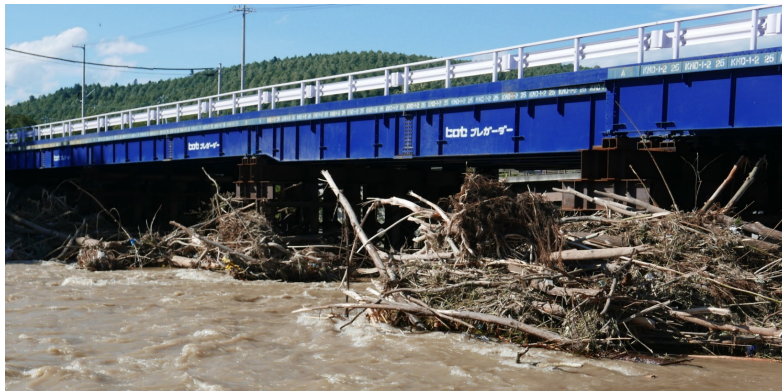
Fig. 9 Accumulation of drift woods on bridges piers of Kiyomi bridge
