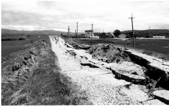
Figure 9 Damage to a dike at the Shiribeshi-toshibetsu river, Hokkaido, Japan, during 1993 Hokkaido-Nansei-oki earthquake
