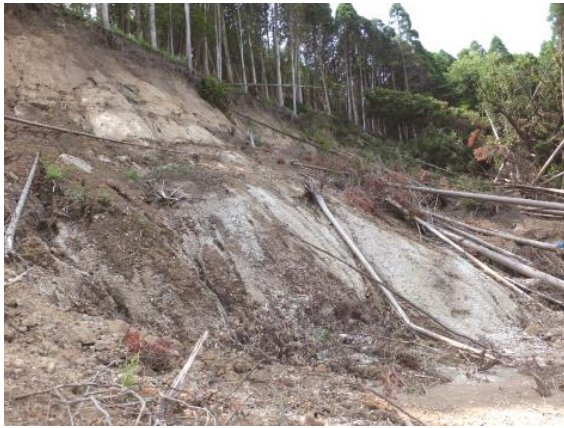
Fig. 41 Oblique view of landslide NGD-3. A sliding surface of Kpfa was widely exposed.
