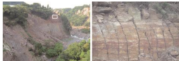
Fig. 6 Landslide of jointed lava on the steep valley slopes along the west side of the Kurokawa River. The right picture is an enlarge picture of the rectangle in the upper picture.
