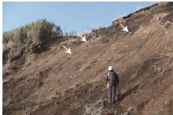
Fig. 27 Oblique view of landslide TKD-1. Arrows indicate the lava blocks.
