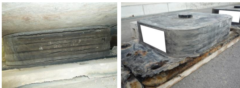
Figure 2.2 Damage status and cracks of ring bearings
