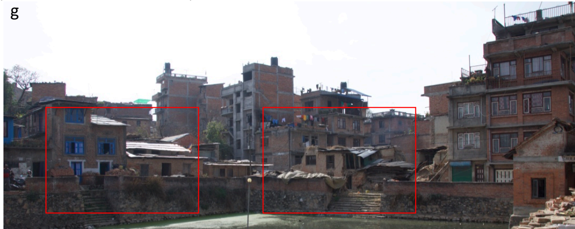
Figure 6.20 g. Photograph of the partially collapsed row houses near De-pukhu taken in 2017 with unsymmetrical openings and changes in the building materials.
