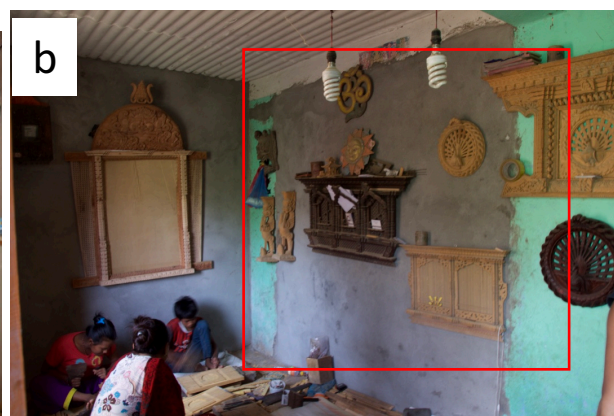
Figure 6.32 b. Damages in the shops which have been patch repaired
