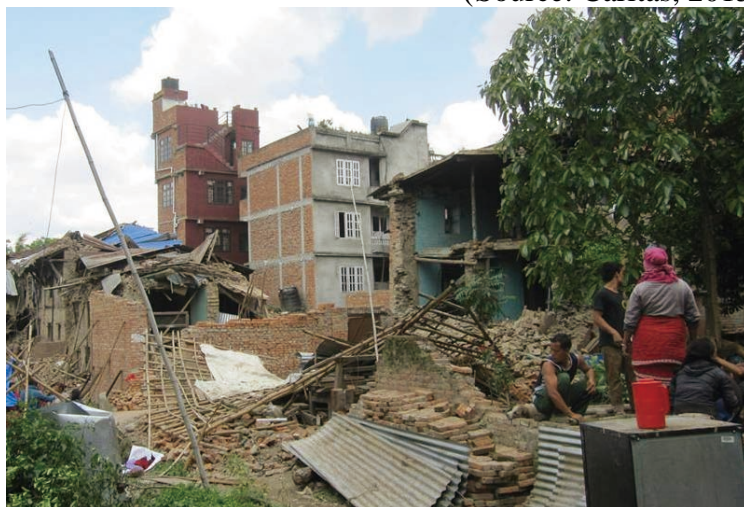
Figure 3.4 Damages to buildings in Bungamati
