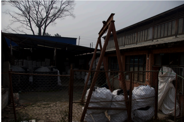
A damaged industrial building in Balaju
