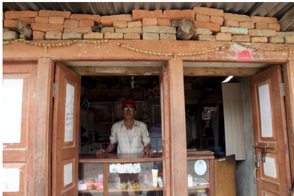
Figure 6.21 c. A tailoring shop running from major damage building in the bus park
