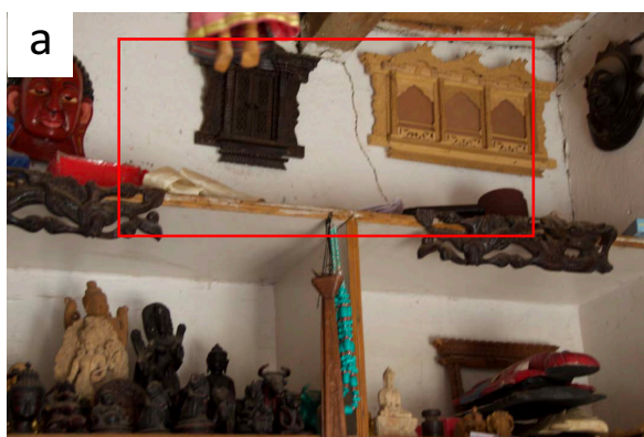
Figure 6.32 a. Damages in the shops which have not been repaired
