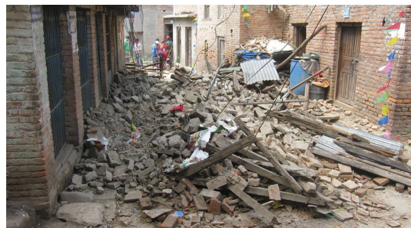
Figure 6.29 b. Street closed due to falling debris
