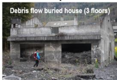
(b) houses in the gully were buried by debris flow
