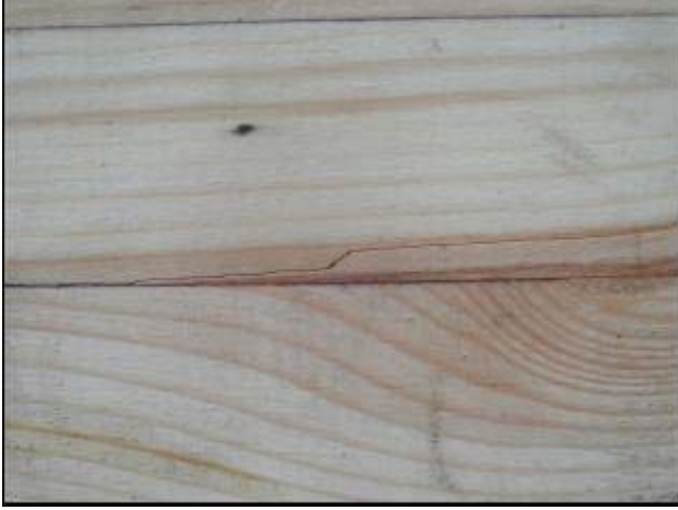
Figure 15 Small scale panel shear failure at the 1 st storey column-beam joint (photo was taken after all test was finished so glulam was laid horizontally).
