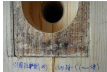
Figure 19 Permanent embedment deformation on the column side surface due to cyclic contact of steel box.
