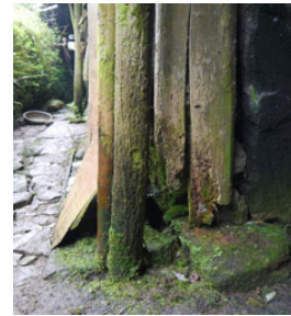
Fig.8 Broken pillar rotten by water
