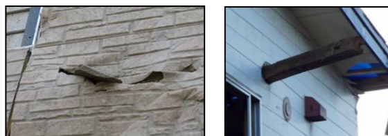
Fig. 1 Damage to houses by flying debris
