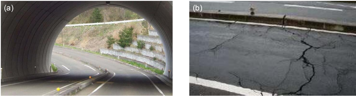
Figure 2.4: Damage to two-hinged arch culvert due to Great East Japan Earthquake: (a) outflow of filling material in apertures of culvert and (b) crack running along pavement.
