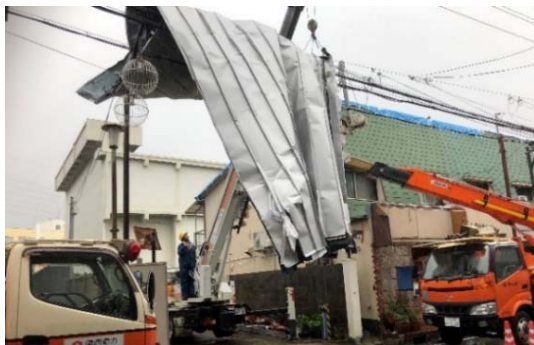
Fig.35 damage due to scattered steel sheet roof (科研費報告書, 2019)
