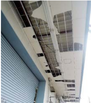
Fig.27 damage to building eaves (科研費報告書, 2019)
