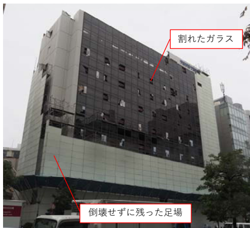
Fig.42 collapse of soundproof scaffolding (科研費報告書, 2019)
