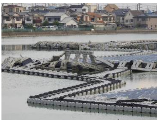
Fig.43 damage to solar farm on a pond (科研費報告書, 2019)
