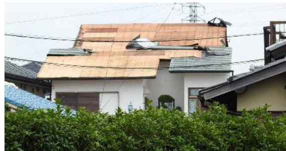
Fig.30 damage and blowing up of roof materials (科研費報告書, 2019)
