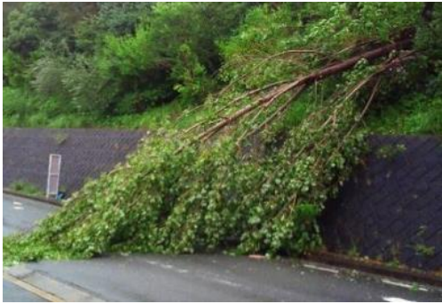
Fig.48 road closure due to uprooted tree (科研費報告書, 2019)
