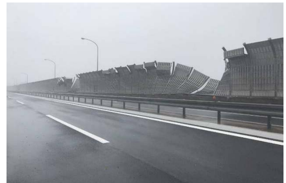
Fig.46 damage to highway sound insulation wall (科研費報告書, 2019)
