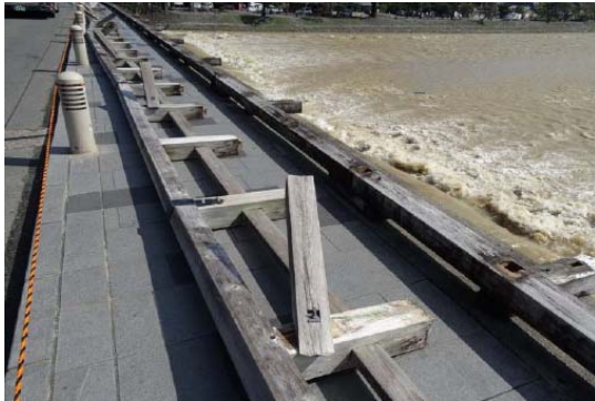
Fig.41 collapse of bridge railings (科研費報告書, 2019)
