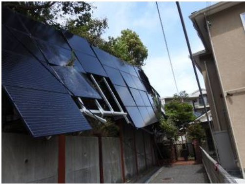
Fig.33 damage to solar panels (科研費報告書, 2019)
