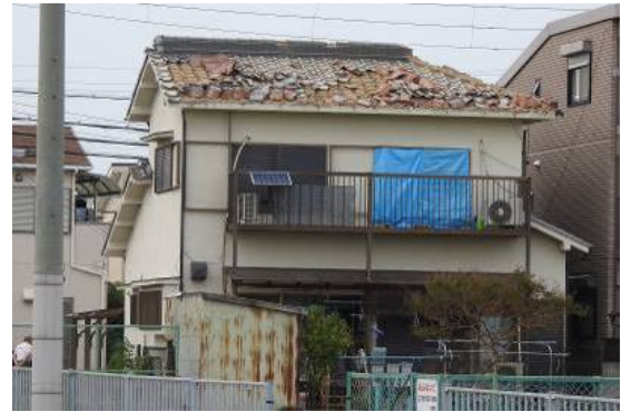
Fig.29 scattering of roof tiles (科研費報告書, 2019)
