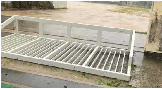
Fig.40 falling of a barricade (科研費報告書, 2019)
