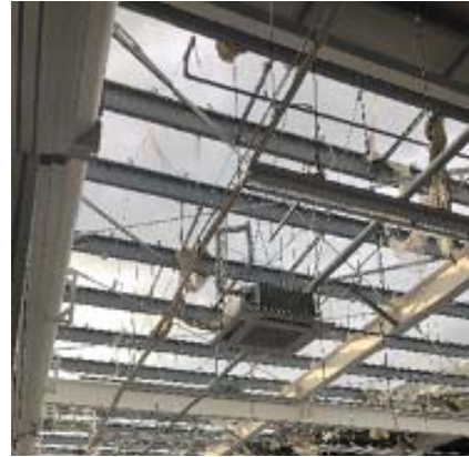
Fig.23 scattered steel plate roof (科研費報告書, 2019)
