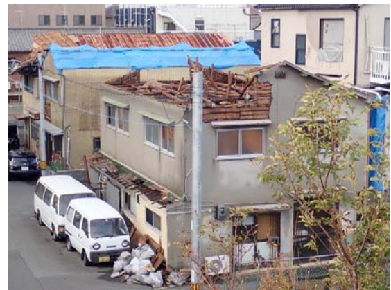
Fig.31 damage to room and loft (科研費報告書, 2019)
