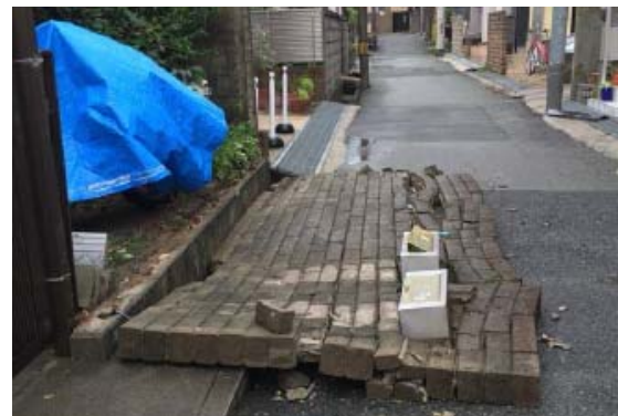
Fig.39 damaged to a concrete parapet wall (科研費報告書, 2019)
