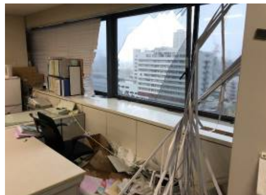
Fig.25 damage to interior due to damage to glass window on the 13 th floor (科研費報告書, 2019)
