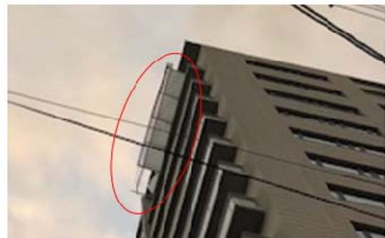
Fig.32 damage to railing of a housing complex (科研費報告書, 2019)
