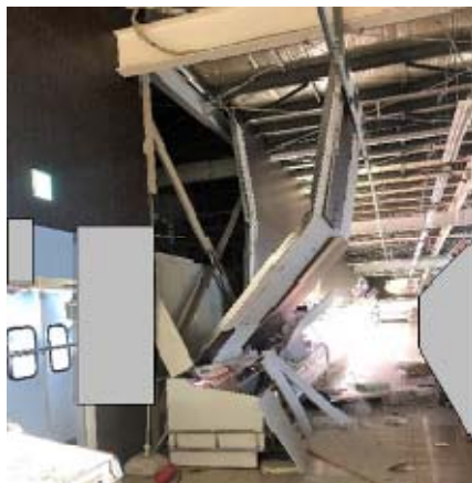
Fig.28 damaged to a store partition wall (科研費報告書, 2019)
