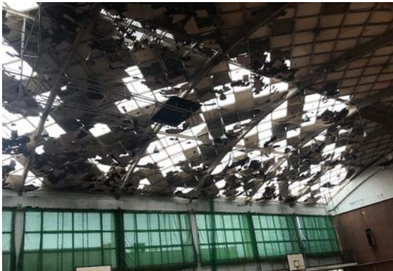
Fig.22 damaged roof of gymnasium (科研費報告書, 2019)
