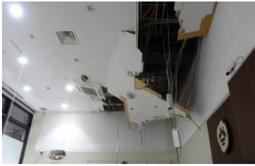
Fig.26 damage to the ceiling (科研費報告書, 2019)
