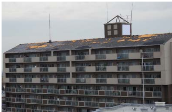
Fig.21 scattered masonry rooftop cladding (科研費報告書, 2019)
