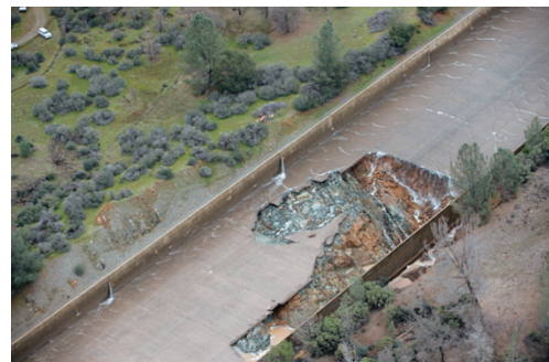
Fig. 2 Oroville dam spillways incident (Matsumoto, 2017)
