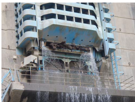
Fig. 1 clogging of outlet of Susobana dam (MLIT, 2018)
