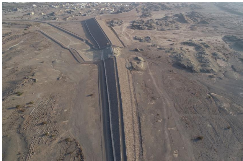
Fig. 6 Al Ameret Heights Dam was taken by UAV, Kyoto University team in 2018.
