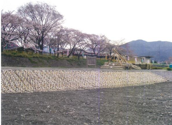
Photo 3 Shore protection using bamboo gabion in the Shimada city (courtesy of Hara Kogumi Co., Ltd.)
