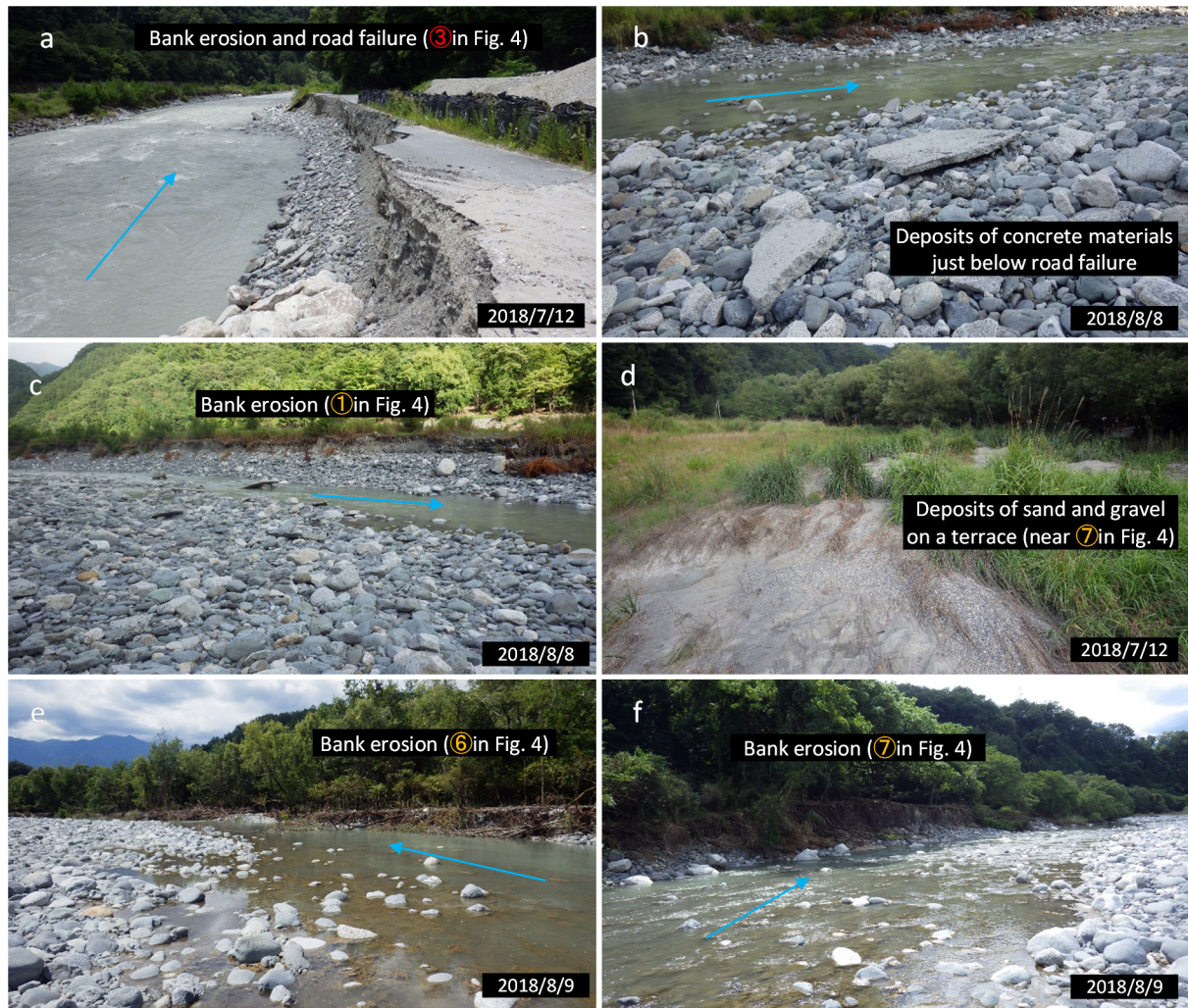
Fig. 7 Photos of bank erosion and sediment deposit
