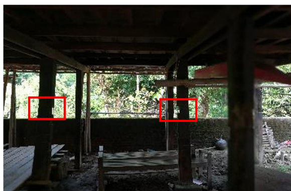
Fig. 4. Marks on the foot pillar for floor elevation since before 2015.
