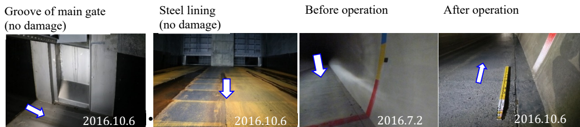
Figure 11: Surface integrity around gates after operation (left) and painted bands (right)
