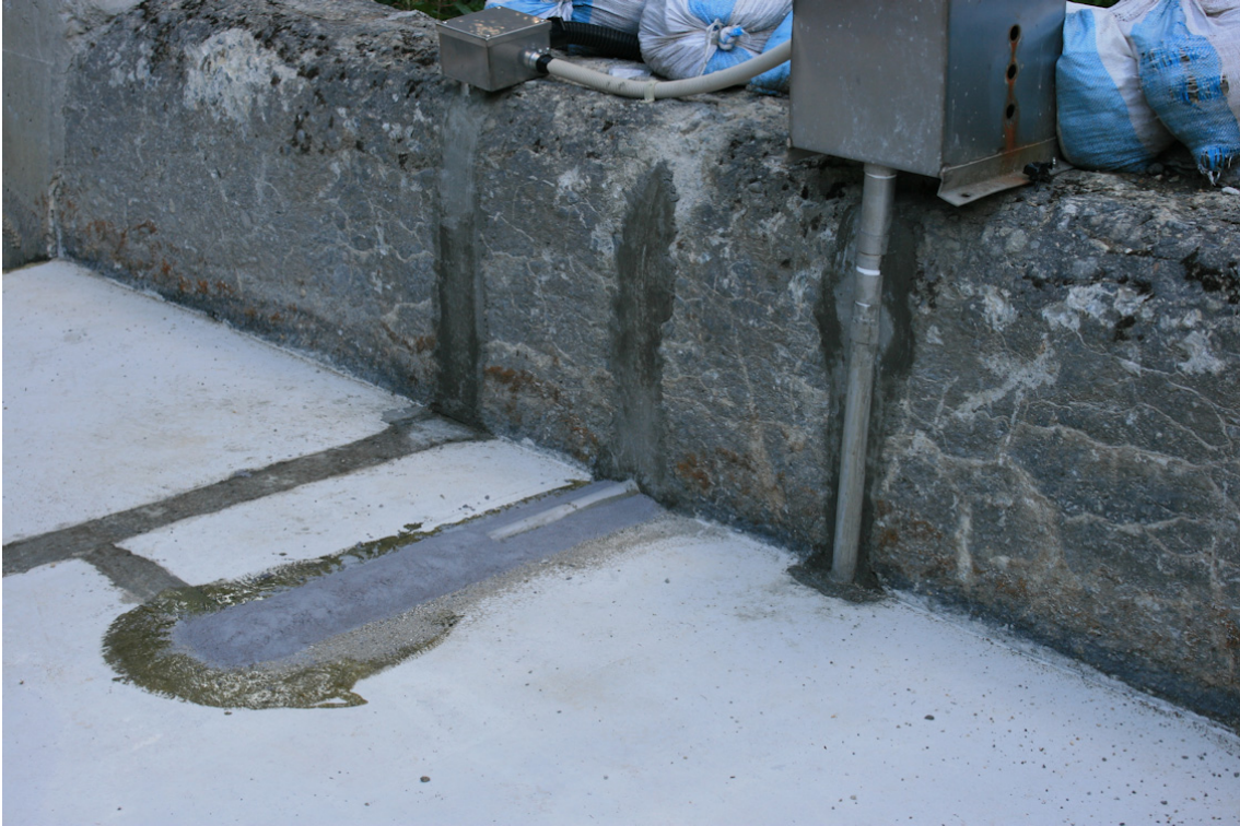
Figure 3: A set consisting of a vertical and a horizontal pipe hydrophone installed at the right side of the Ashi-arai-dani flume.
